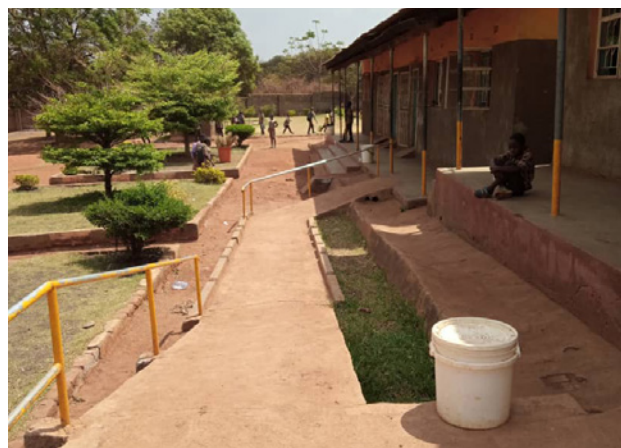
Inclusive education requires a school to be accessible for all. Thanks to maintaining enduring relations with external stakeholders, ramps and handrails were constructed.
